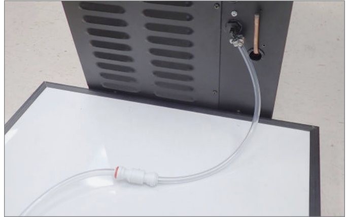
FIG. 5. Installed check valve.
