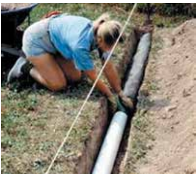
Figure 71: Underground Refrigerant Piping.
