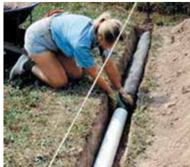
Figure 71: Underground Refrigerant Piping.
