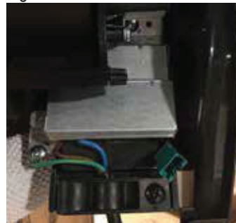
Figure 84: Terminal Cover Down.
