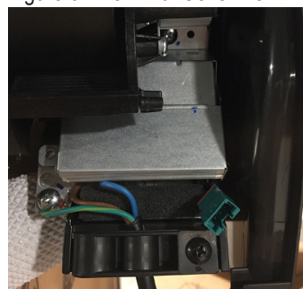
Figure 82: Terminal Cover Down.
