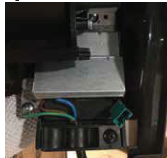
Figure 84: Terminal Cover Down.
