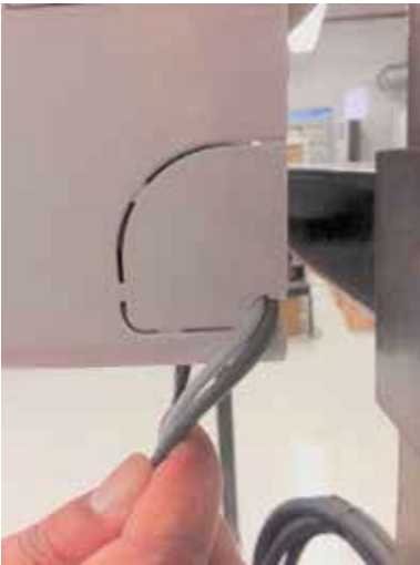
Figure 90: Indoor Unit Knockout (Communication Wires)
