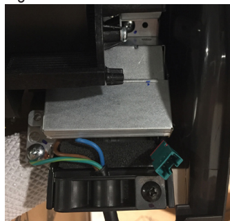
Figure 82: Terminal Cover Down.
