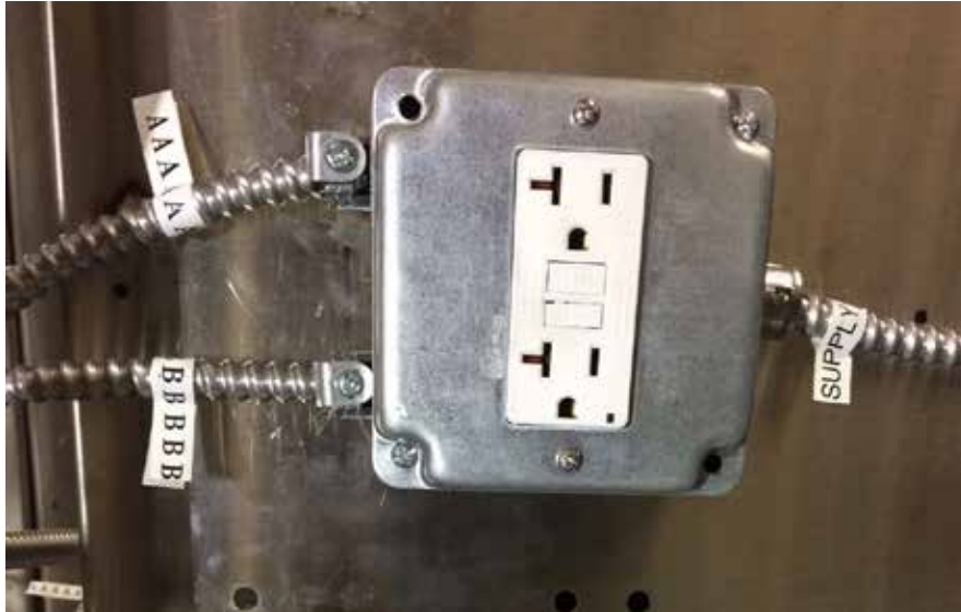
MAIN ELECTRICAL BOX COMPLETE
