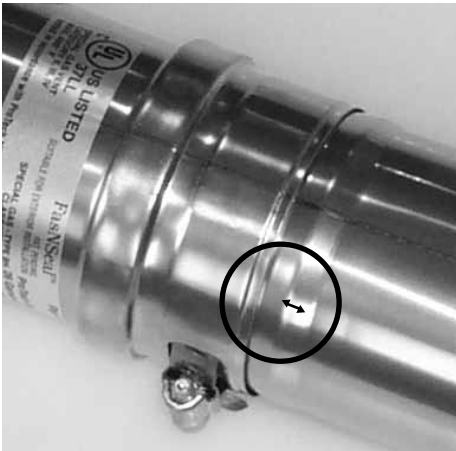
INCORRECT Joint Connection. Male/Female sections NOT fully engaged.
