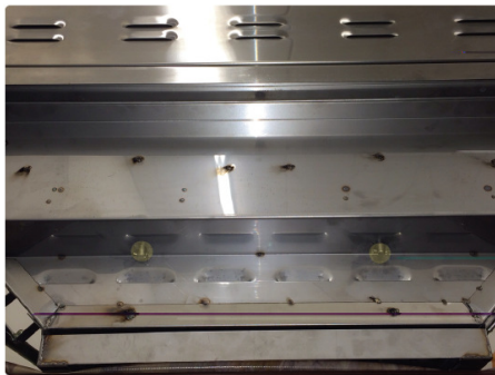
Cotter pins holding burners in place
