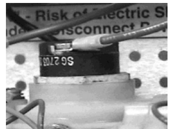
Figure 11: Installed heating element
