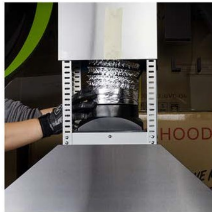
22. Secure the inner chimney cover to the ceiling plate with the included screws.
