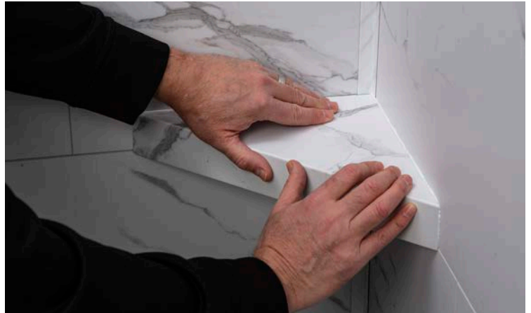
Wipe off any excess sealant that pushes out or add sealant in areas needed.
