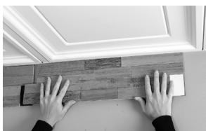
Moving left to right, use overlap notches to abut tiles, just as you would in a backsplash installation.
