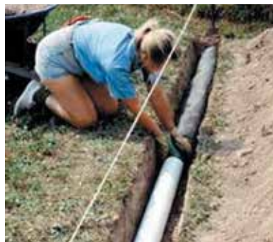
Figure 71: Underground Refrigerant Piping.
