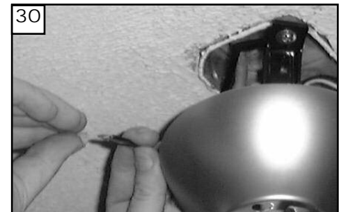
30 Make wire connections to power source using wire nuts provided. Make sure that no filaments are outside of the wirenut. After making the wire connections, the wires should be spread apart with the grounded conductor and the equipment-grounding conductor on one side of the outlet box and ungrounded conductor on the other side of the outlet box.
