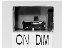
Left side of wall control
