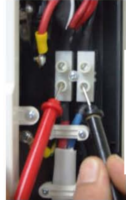
Measure voltage from L1 to L2 Should get 208/240
