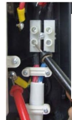
Measure voltage from L1 to Ground. Should get 110-120
