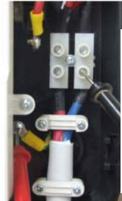
Measure voltage from L2 to Ground. Should get 110-120
